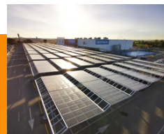
PV CARPORTS DECATHLON
